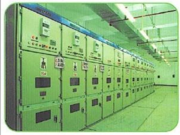
Voltage switch system
