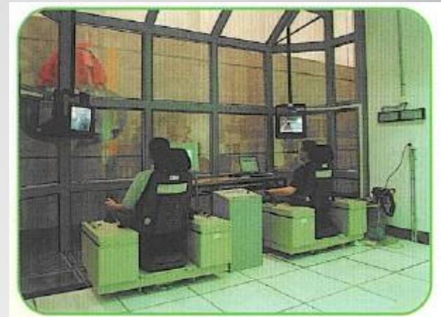
Refuse crane control room
